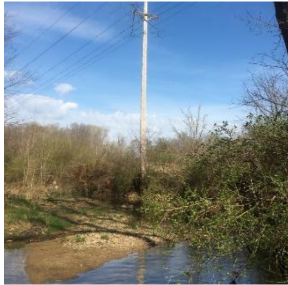
FIGURE 2-10: EXPOSED BASE OF POWERLINE POLE AND ERODED STREAMBANK
